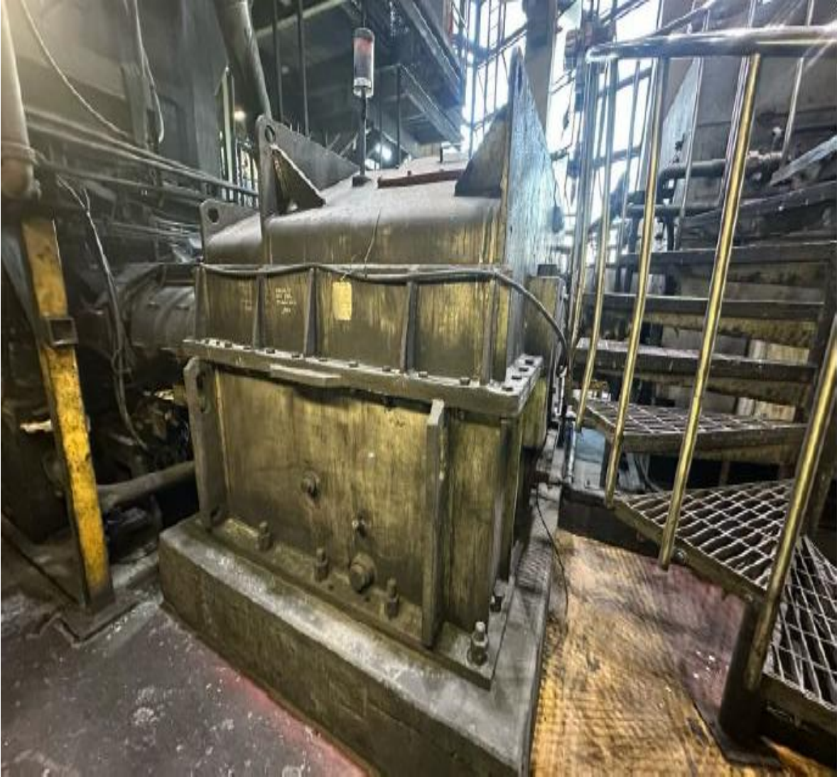
Figura 18. Motor reductor principal Mixer 5
