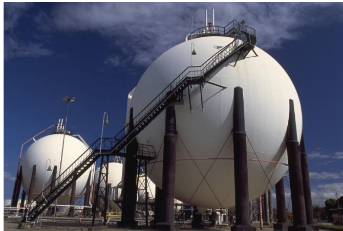
Figura 4: Estanque esférico GLP - https://c2.staticflickr.com/8/7229/7403662710_4f7b5d7bdb_b.jpg
