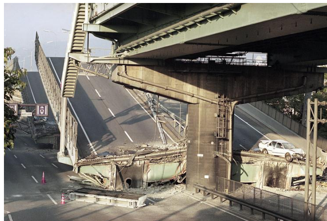
Figura 2: Colapso del Hanshin Expressway, terremoto de Kobe (1995).
