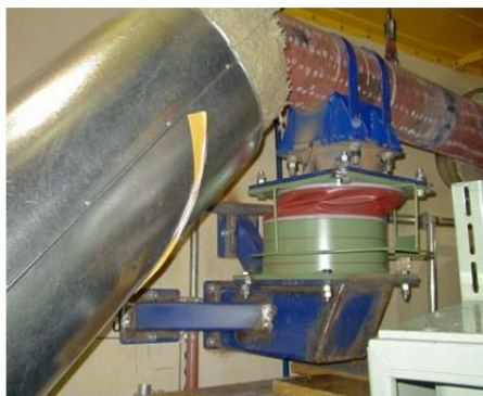
Fig. 8 VES damper at the RL76 in RB LO2 (damper's piston at the piping, housing at the RB wall)
