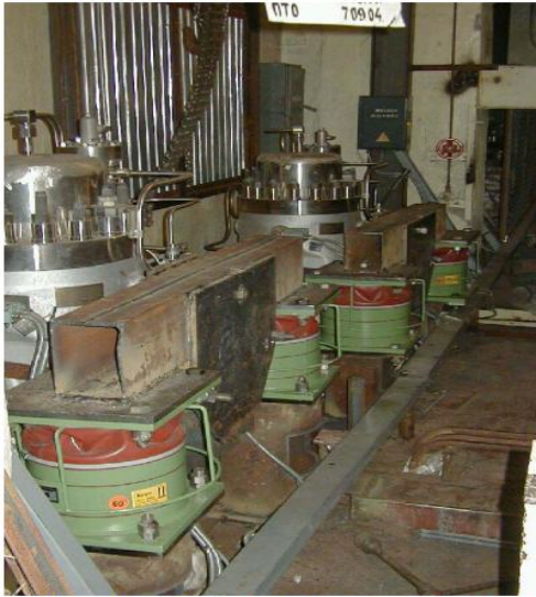
Figure 7. General View of the Dampers on the SEBIM Valves 1211 (front) and 1234.
