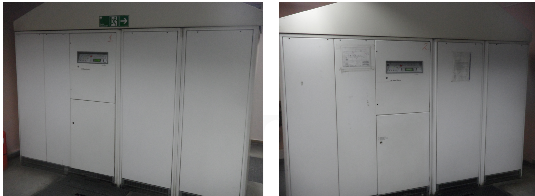
(a) UPS N°1 General Electric 250 kVA
