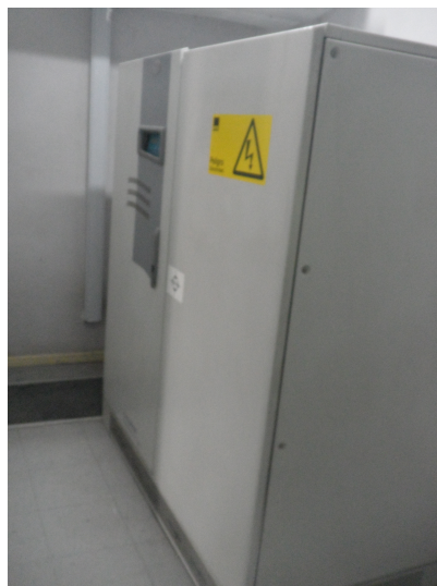
(a) UPS N°1 Chloride 250 kVA
