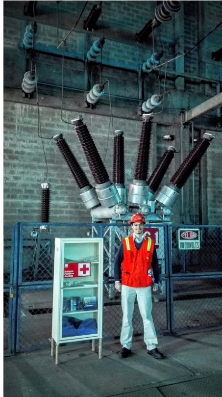
Figura 2.2: Interruptor central Tocopilla, I_k :40kA, I_n :1200A, V_n :123kV .
