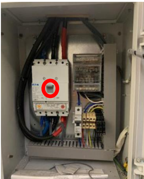
Figura 25: Interruptor tablero principal.
