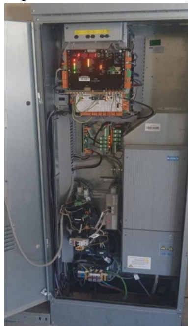
Figura 2.9: Gabinete de control
