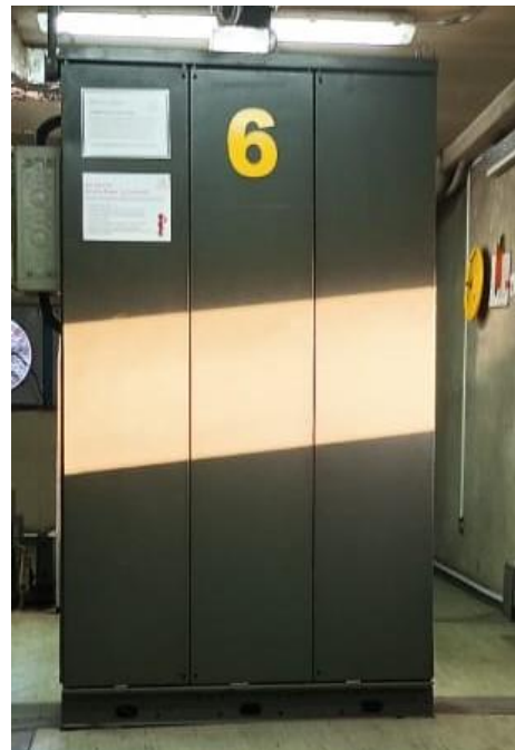
Figura 2.4: Gabinete de control
