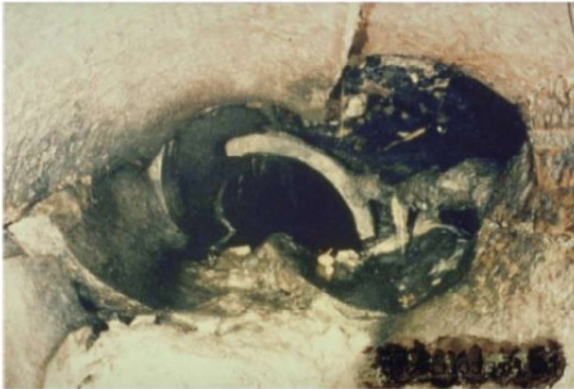
A-11 Colapso (X)
