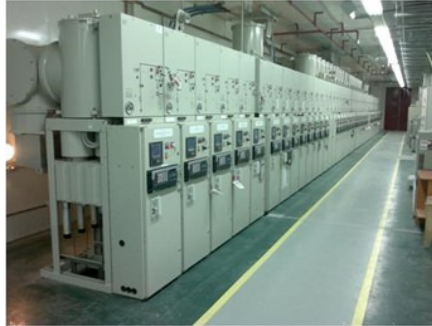
Ilustración 3: Vista Switchgear S/E Principal CMDIC 23 [kV]
